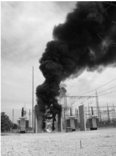
Figure 7. Fire Plume from a Reactor Fire
