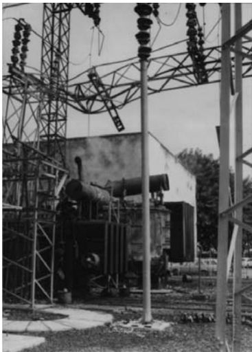
Figure 2. Impact of A Transformer Fire on A High Voltage Bus Structure
