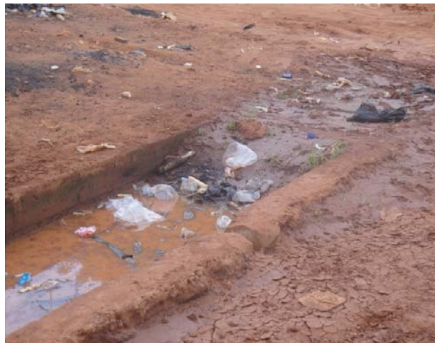
Plate 2: Blocked Drainage Along Old Egume Road
