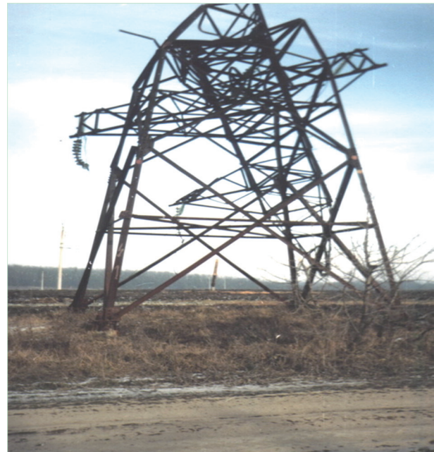
Figure 3 Reliance, Collapsed Under the Weight of Ice
